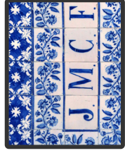
14 Recently restored building, its original tiles were replaced with replicas. The photo dates back to 2015 containing the original tiles. The monogram corresponds to the name José Marques da Costa Freitas (J.M.C.F.).
